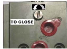
Manual Override "ON" Photo - 3
