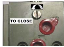
Manual Override "ON" Photo – 3
